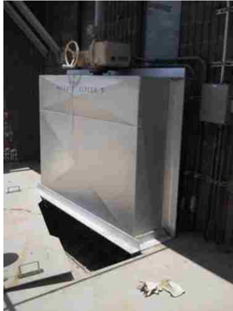
Figure 26 Gate Cover and Plate Over Effluent Channel
